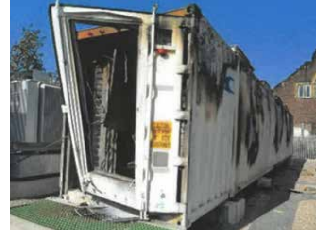
Above: Test case Battery Energy Storage System, destroyed by thermal runaway event occurring in lithium ion batteries.
