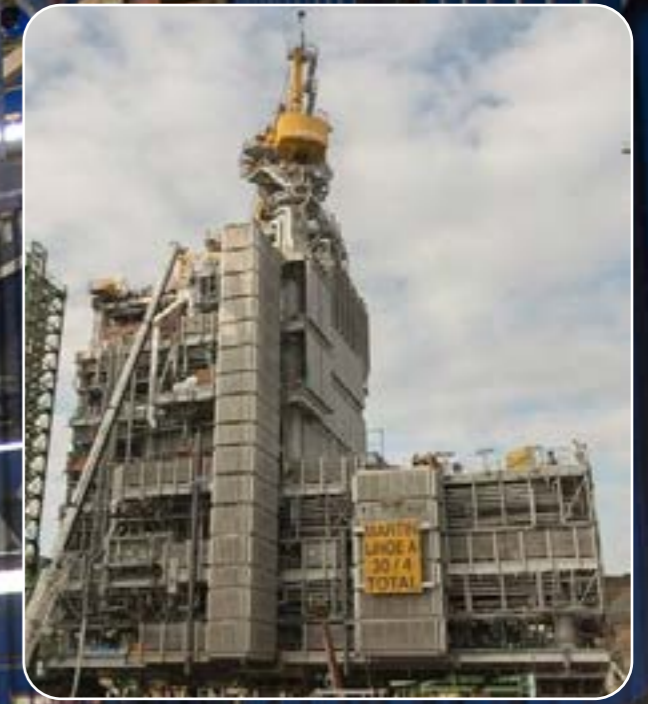
Above - Martin Linge Stair Tower and Walkway Heat Shields
