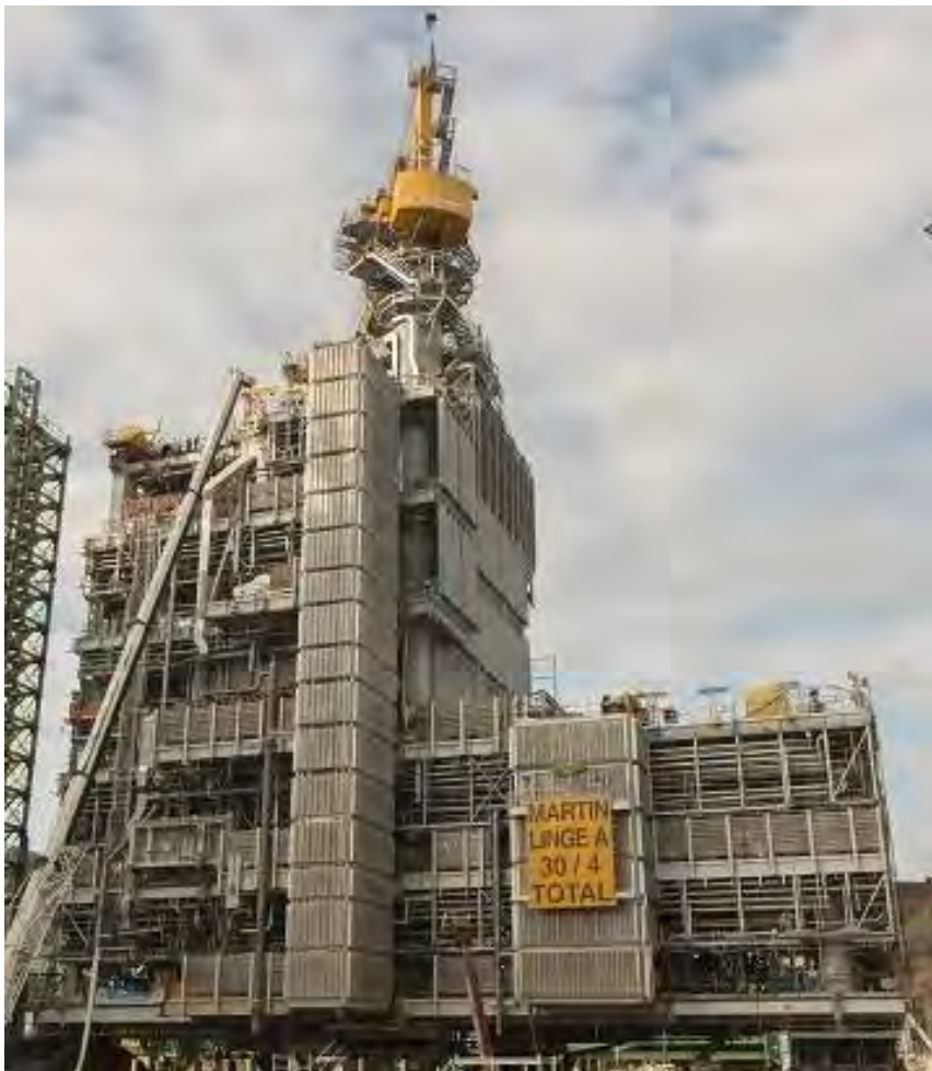
Martin Linge – Stair Tower & Walkway Heat Shields
